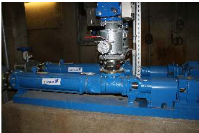
Approximately 80% of all pumps in the plant are from Allweiler®, including the thin sludge pumps in this photo.
