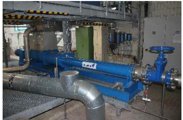
Four-stage solid-substance progressive cavity pump, type AE4N1450-RG from Allweiler®, used as residual sludge discharge pump, below the centrifuge.
