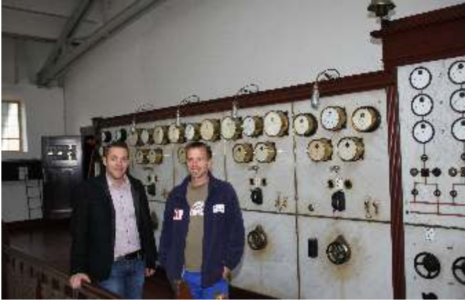
A portion of the early control panel.
